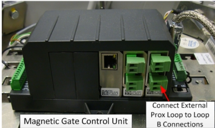
Figure 27. Magnetic Gate Control Unit
